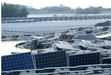
Damaged floating-type solar power generation facilities in Ichikawa City, Chiba Pref. (Due to a typhoon in September 2019)
