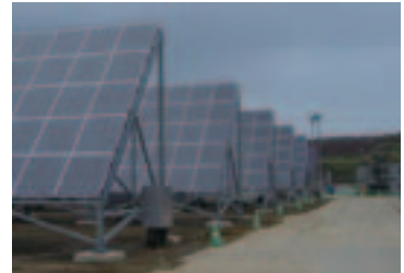
Mega-solar Wakkanai Site (Wakkanai City, Hokkaido). Project contract: NEDO.
